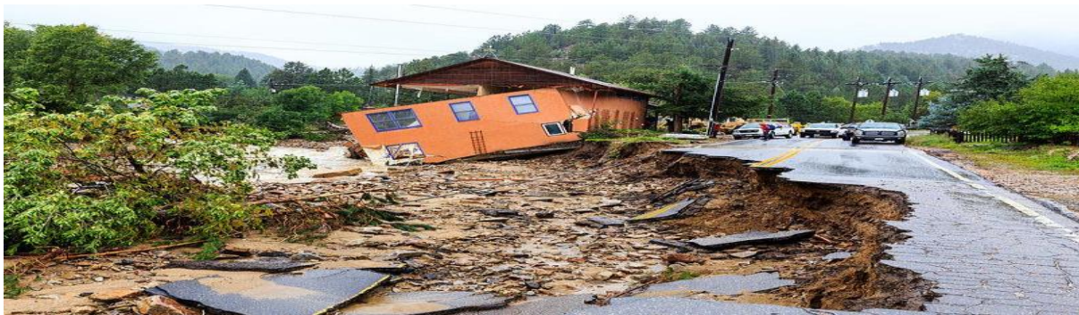
Image 3: Damage Due to Flood
