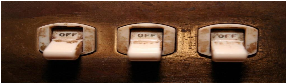
Image 7: turning off electrical switches
